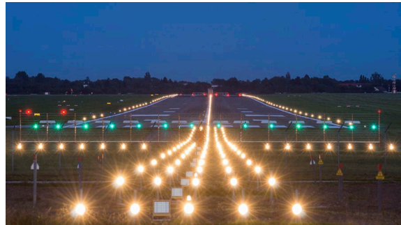
Airport – runway lighting www.stantec.com
