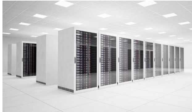
Data Centre Power Outage Image: https://powerwhips.com
