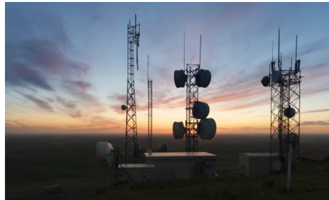
Telecommunication facilities www.securitysales.com/
